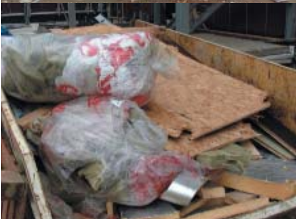
Unusable Rockwool offcuts
